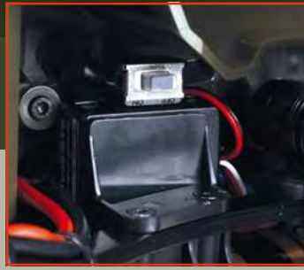
Although the electrics are tucked neatly out of sight, the switch is easily accessible
